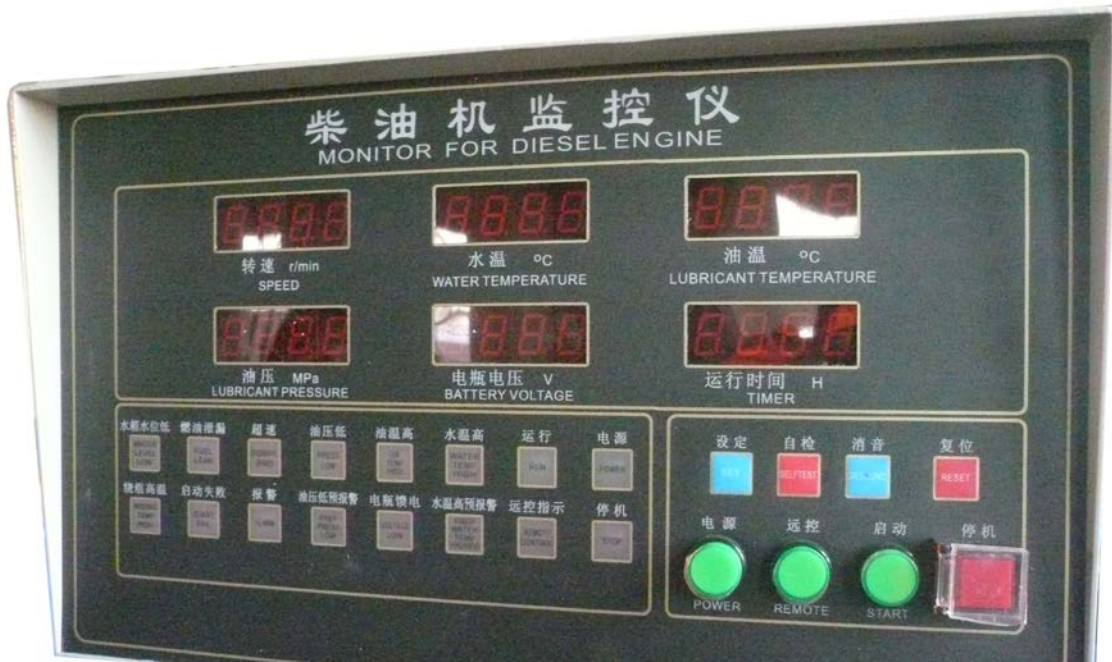
Engine control panel
